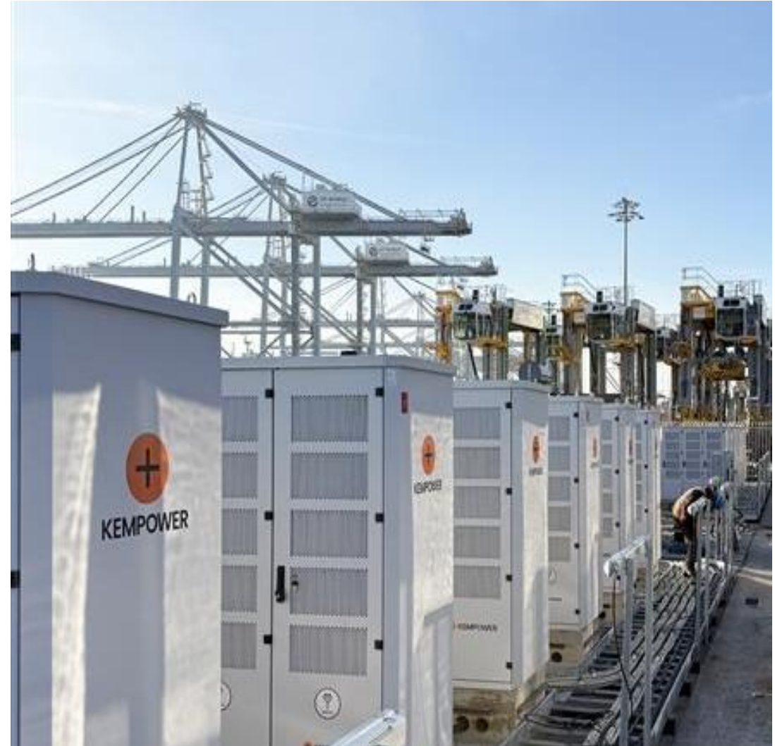
Photo: MCS chargers at DP World's port in London Gateway
