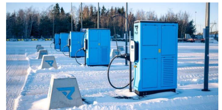
Photo: Plugit's first public MCS charging station in Kotka, Finland
